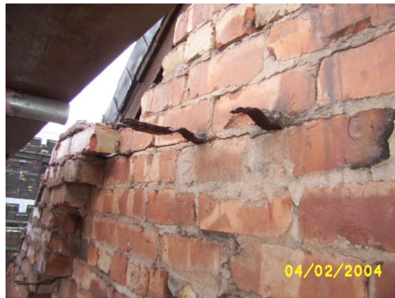
Corroded thick metal ties where outer leaf has been dismantled
